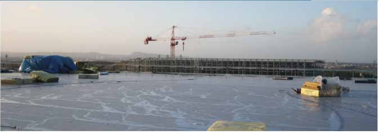
Portugal , Setubal, Portucel plant, 11.000 m 2
